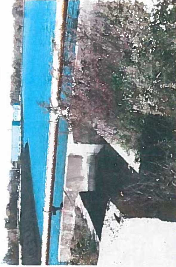
Photo Number: 3 Date of Photo: 10/17/12 Description: Looking north at Ash Surge Basin inlet structure. Creator: JRR
